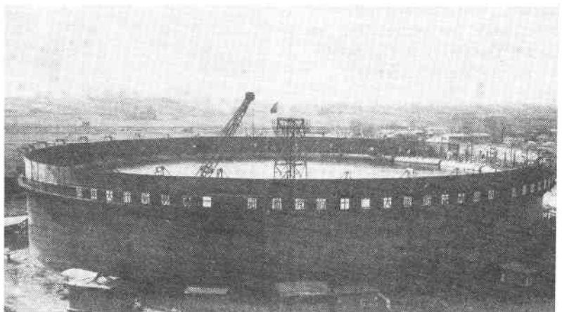
China's biggest gas storage tank is being built in Beijing which will improve fuel supply and reduce urban pollution.
