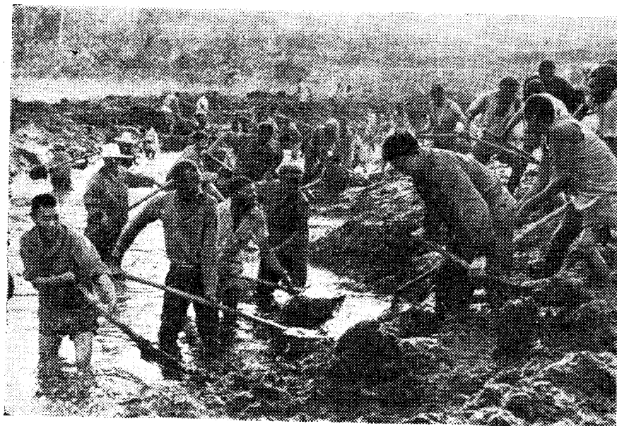
Chinese personnel and Zambian workers drain marshy land to build the railway.
