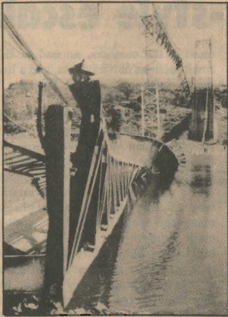
Twisted wreckage is all that remains of the Cuscutlan Bridge destroyed by the Salvadoran revolutionaries.
