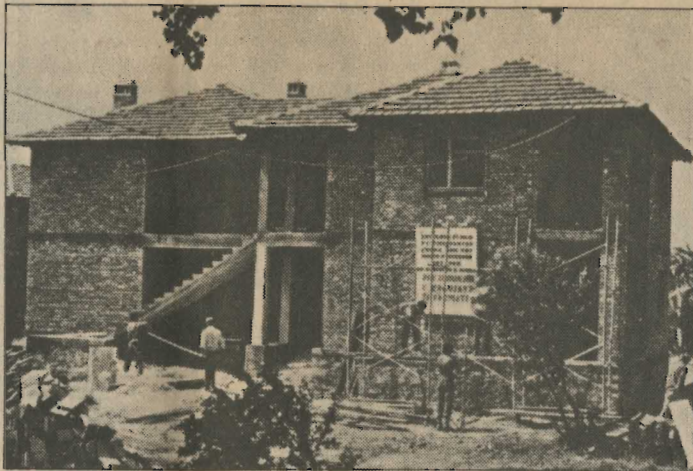
completely rebuilt. The two above photos show the working masses beginning the rebuilding process and new homes almost completed.
